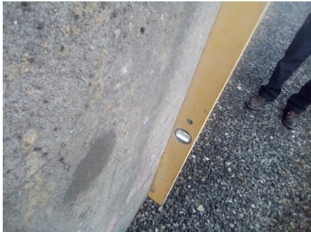
Out of plumb shift
