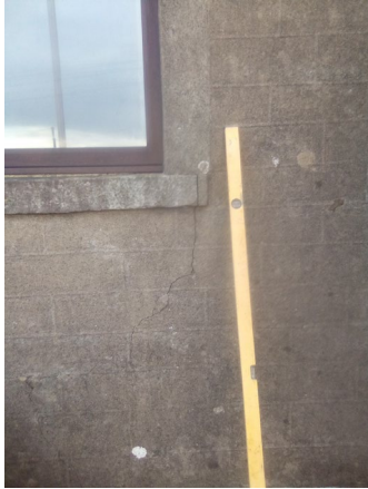
Crack at window cill
