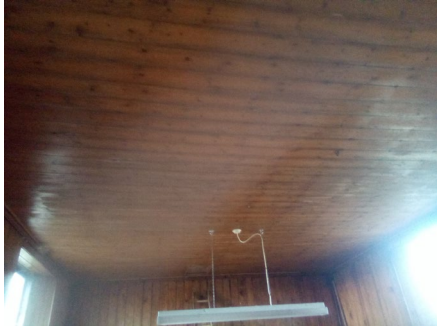
Significant sag in ceiling
