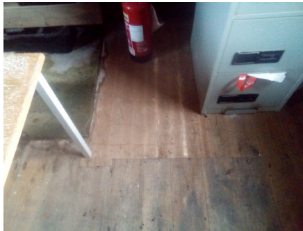
Wood dust on flooring
