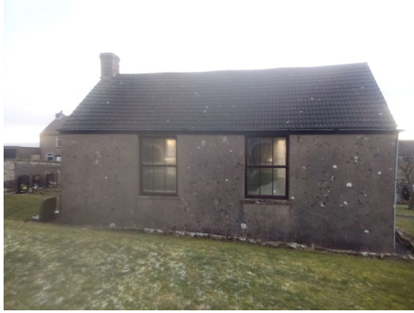
Ridge line uneven
